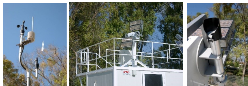
Two axis tracker / solar irradiance assessment
